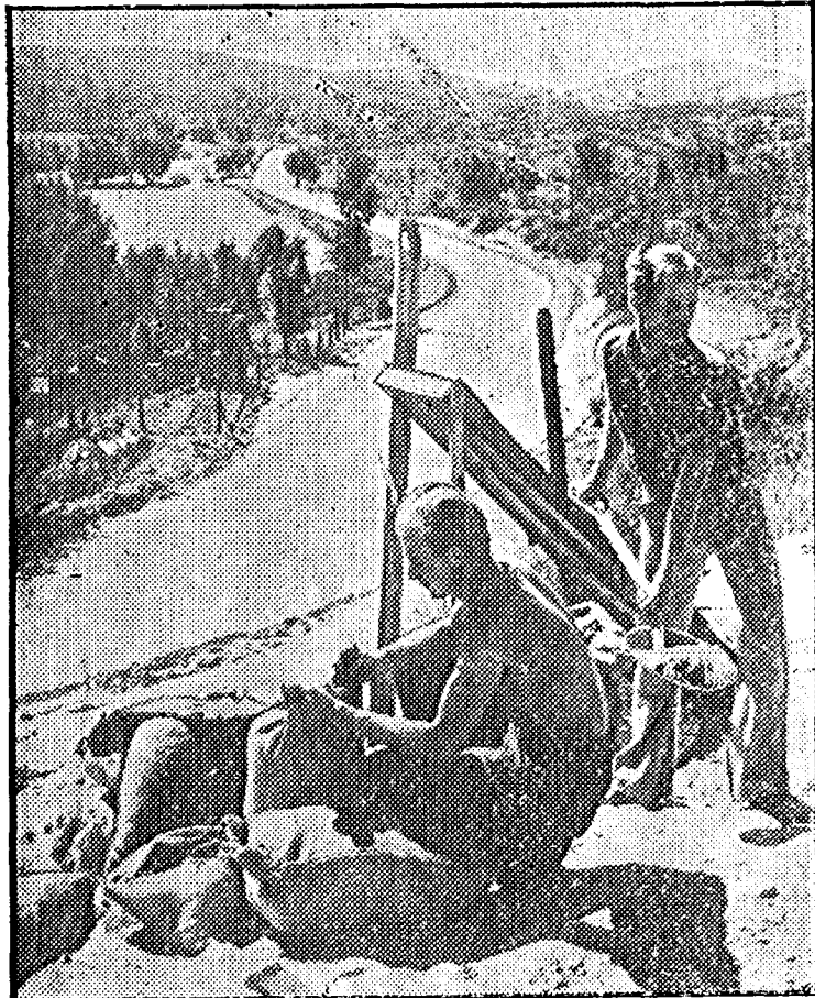
Connecting Julian and Ramona, Calif., in the heart of San Diego county's mining region, this highway is literally paved with gold. Constructed in 1926, it was found recently to assay $7 a ton. Material for the road was obtained from a quarry, and Fred Koelke and Orval Hammer are shown here searching for gold-bearing quartz on the quarry dump. County supervisors said it would not pay to tear up the road and sell the ore.
