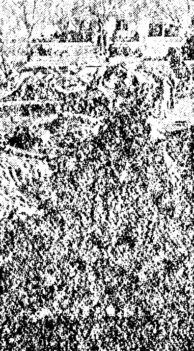
Clausen & Sons' big dragline is making short work of the excavation for Ord's new swimming pool now being built at Bussell Park. Work will progress rapidly once dirt moving is finished. — Swopes photo.
